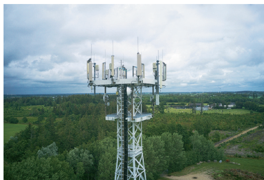
Fig. 1. 5G towers like this one are now transmitting at frequencies that are close to the frequencies used by aircraft altimeters. Expanding service to these frequencies offers better performance for cell phone users but could interfere with the proper functioning of some altimeters. Credit: Fabian Horst (CC BY-SA 4.0).
